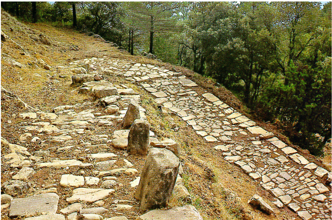
Figure 25, The technologically poor Capsacosta road, in Gerona. An unengineered mule track, claimed and presented as Roman
