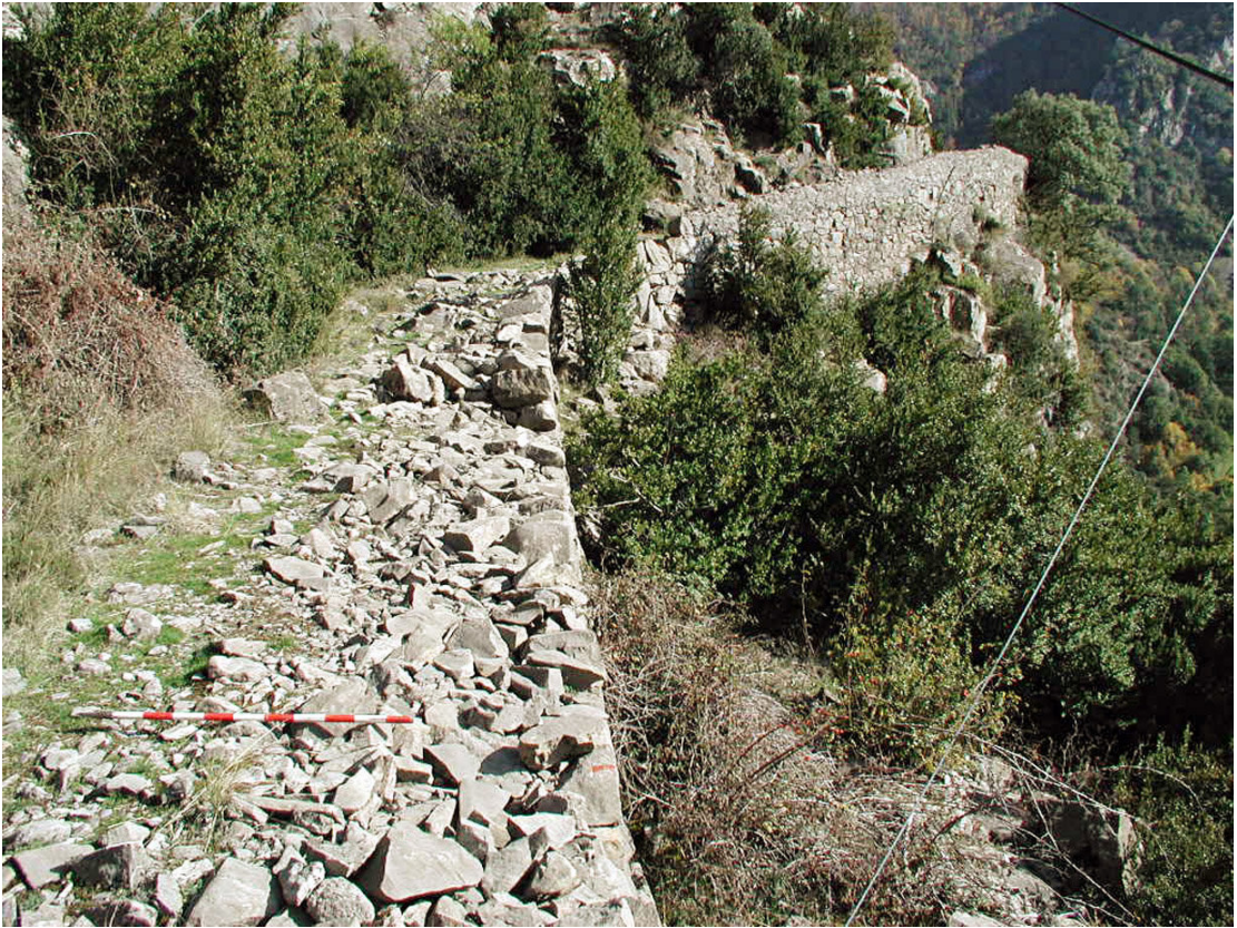
Figure 26, View of the Puerto del Palo road at the only site with any constructive structure of interest. It is a poorly made retaining wall to support a two-metre wide path. Cuellos de Lenito in the Valle de Echo
